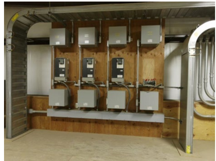
VFDs for cooler motors – in the mezzanine above the control room
